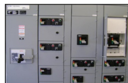
Motor Control Centers
