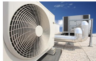
Air Conditioning & Spares
